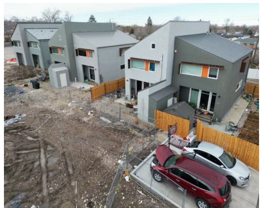
March 10, 2023. Right to left: four occupied homes (with 11 children), two under construction.
